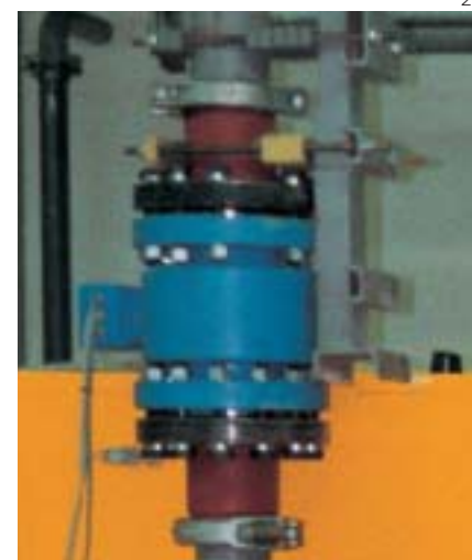
Inductive metering of pumping output
